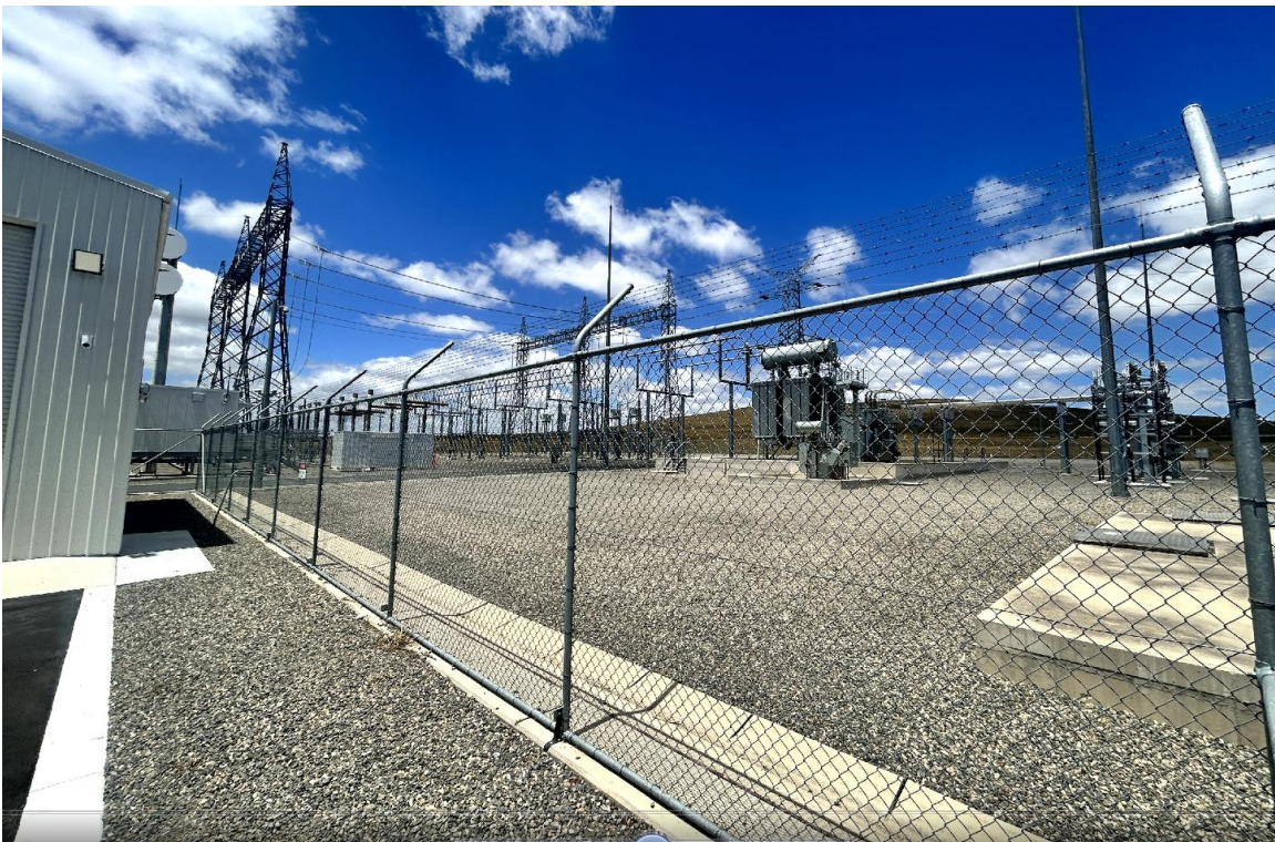
Figure 16: High resistivity surfaces in and around the Control Room and substation
